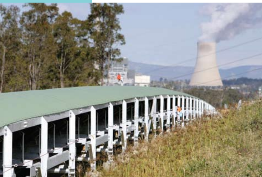
Part of the 5.5km conveyor connected the unloader to the Bayswater Power Station.
